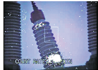
(a) 套管微裂纹
